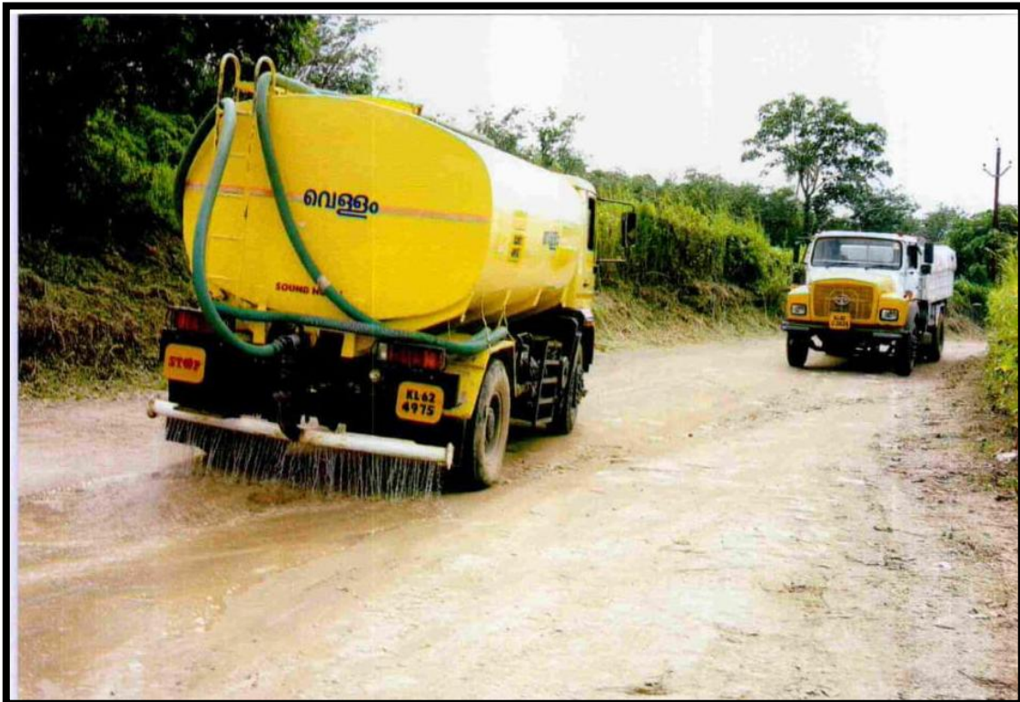
Water tank with sprinkler
