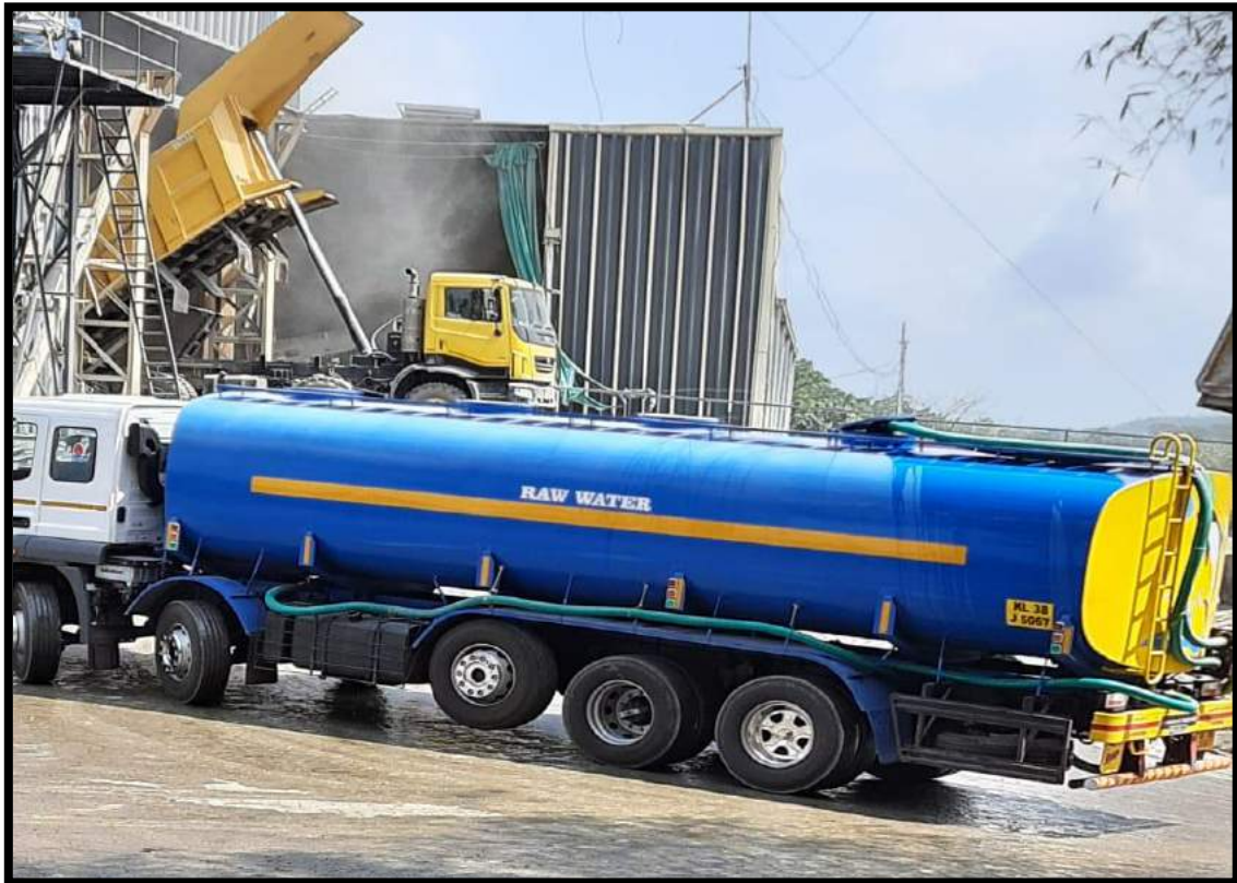
28 KL Water tank with sprinkler
