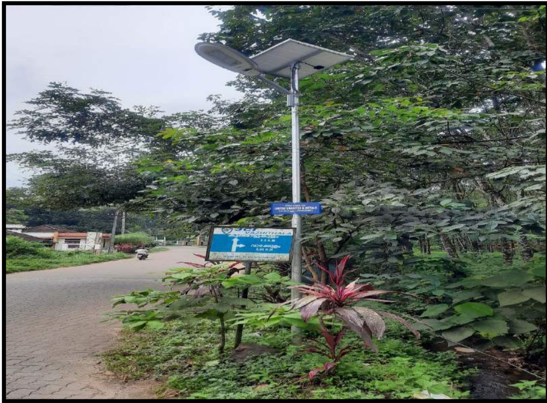
Solar light installed in public road
