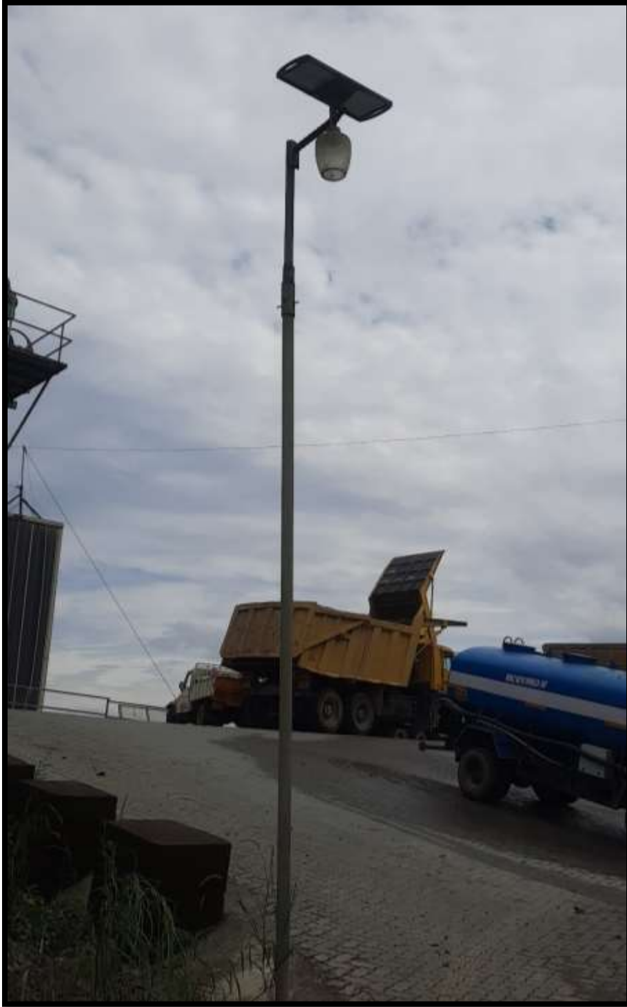
Solar Lights installed at the site
