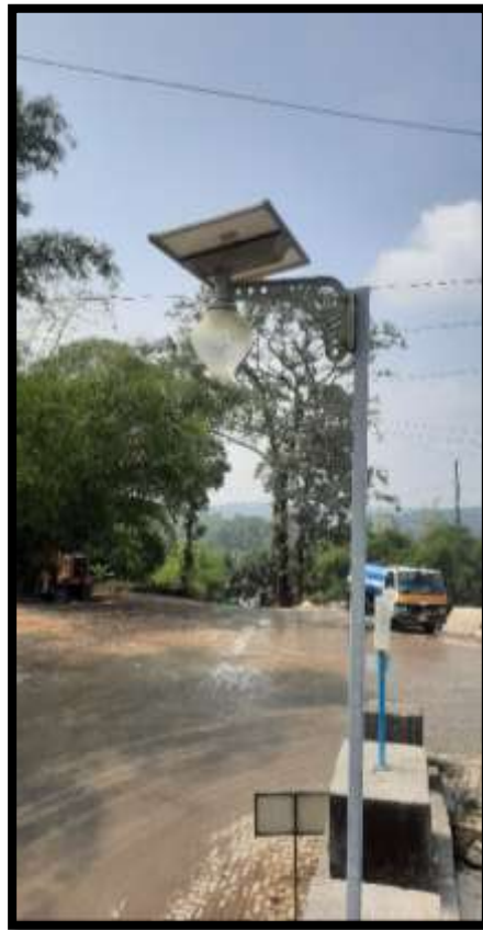
Solar Lights installed at the site
