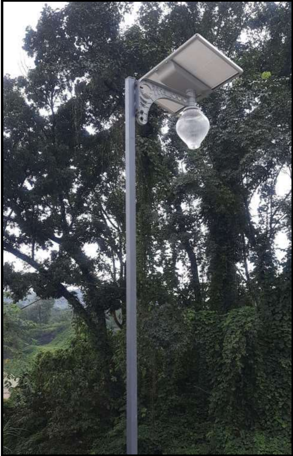
Solar Lights installed at the site
